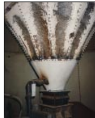
"Hammer tracks" show this hopper has chronic—maybe terminal—bridging problems.
