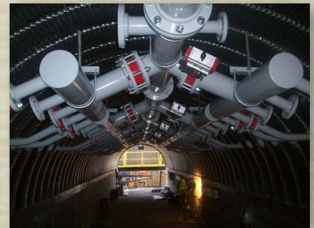
PLC-controlled air manifold system in the access tunnel delivers clean air from the blower system to the air-gravity conveyors.
