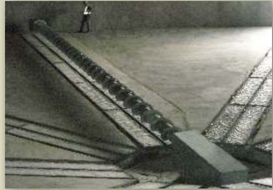
The reclaim screw is parked at a "home position" over any one of the air-gravity conveyor spokes prior to fill.
